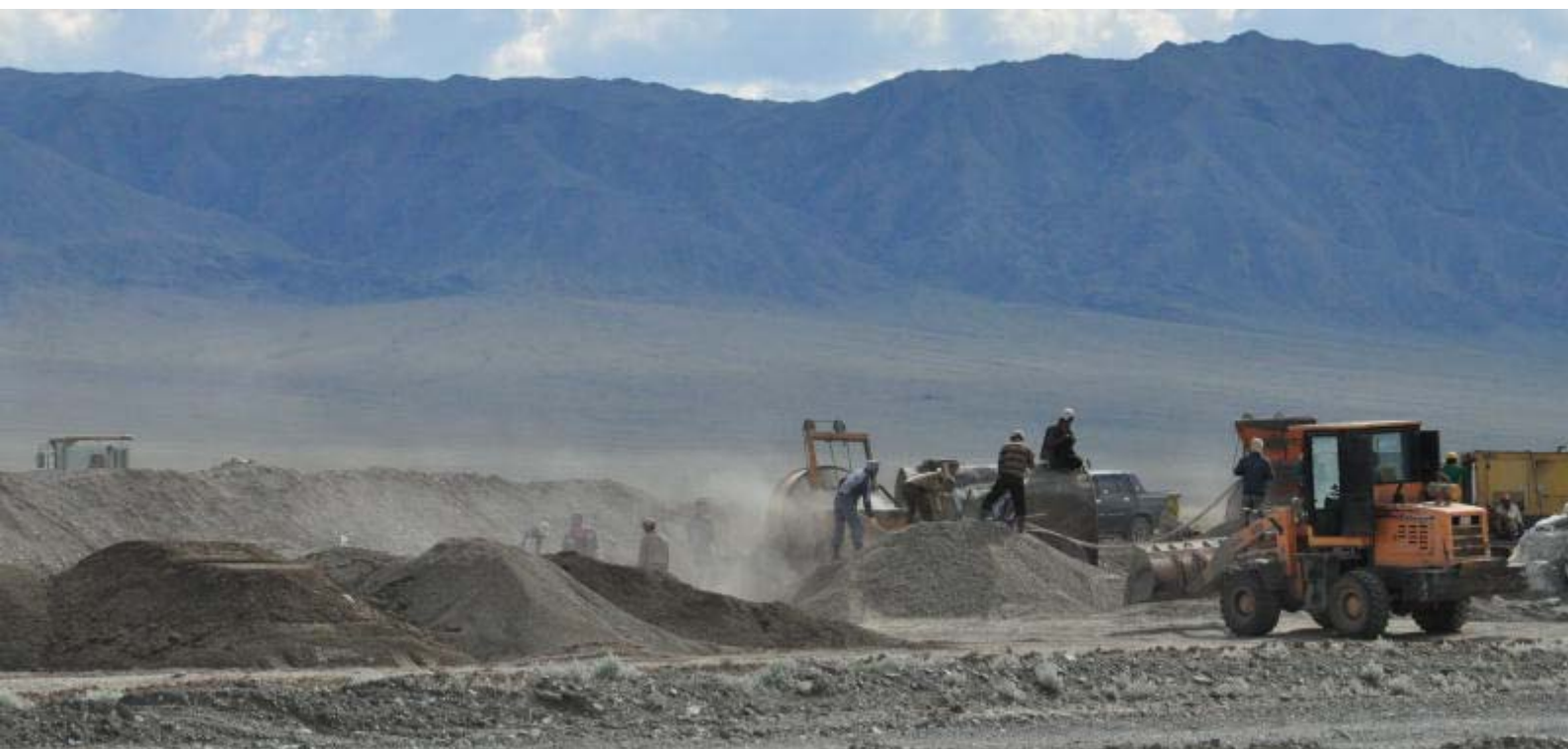
Construction site of the new black top road. The steep mound of the road can be seen in the background on the left.
